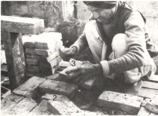
345 The brick layer cutting the brick to size with his axe (dājyācupi).
