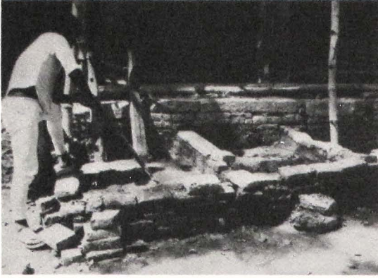
360/361 Preparation of bajra for the restoration of the Gārath-ghar palace in Nuvākoṭ (1983):
