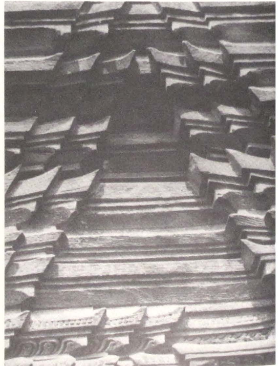
592 Bhaktapur: Dhaubhadel house of Taumādhi, 18th cent., kulā-design of the secondary lintel (below with palehaḥ-lotus leaf and pū-bead pattern), lintel (middle) and cornice (above).
