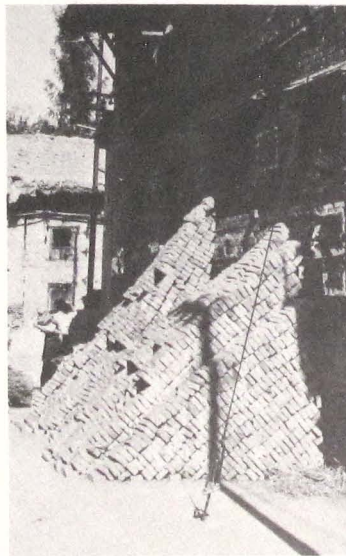
212 Support of a wall by a pile of bricks serving as an abutment.
