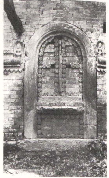
495 Godāvāri: Pulcokimāi; door in the enclosure wall filled with moulded bricks, suggesting an apron and door leaves.
