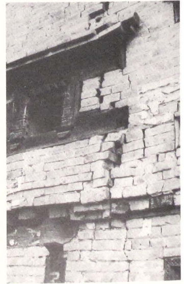
213 Cracks signalling insufficient bondage.
